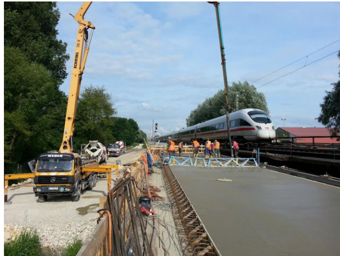
Permanent way concreting M-IN of the rail overpass pair for construction phase 18.3
